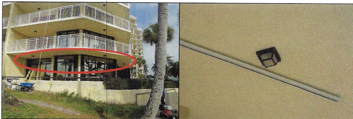
Figure 10: Photo of the existing ceiling mounted fixtures on the south facing ground floor level, circled in red, and a close-up of a ceiling mounted fixture.
