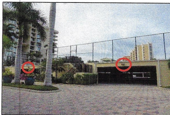
Figure 3: Photo of the existing wall packs on the south facing carport entryways, circled in red.
